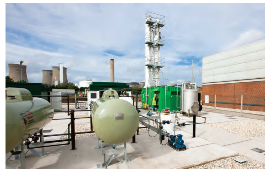
The Chesterfield BioGas upgrader at Didcot, the UK's first plant producing biomethane for injection to the national gas grid.
